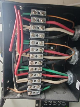
Spare Transfer Switch carried onboard: WFCO T57 50 Amp – Purchased Aug 23, 2022
